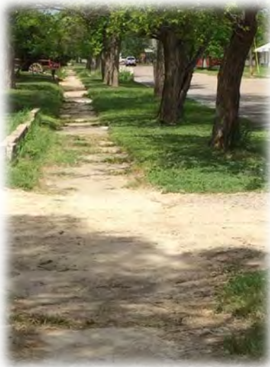
Sidewalk Covered with Soil and Grass
