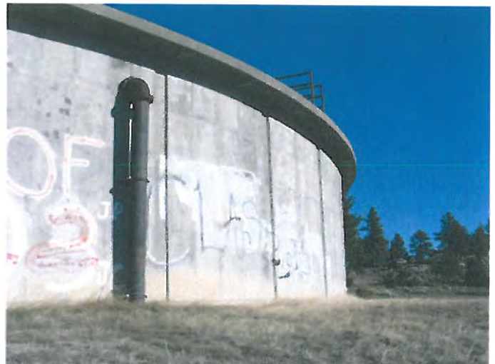
Storage tank overflow pipe and portable ladder access point to upper hatch and vent (ST001)
