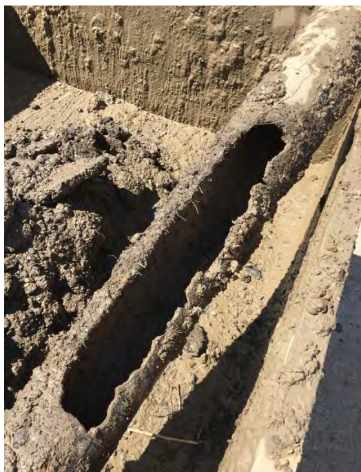
Figure 3.8: Section of Burst Cast Iron Water Main
