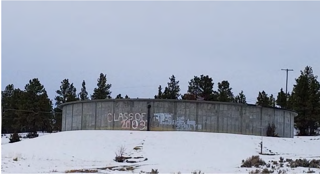
Figure 3.4: Ground Level Water Reservoir
