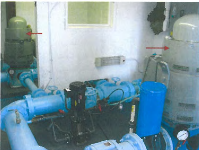
Pumps for the two wells completed in the flooded Republic #1 coal mine (Inventoried as one source, WL003)
