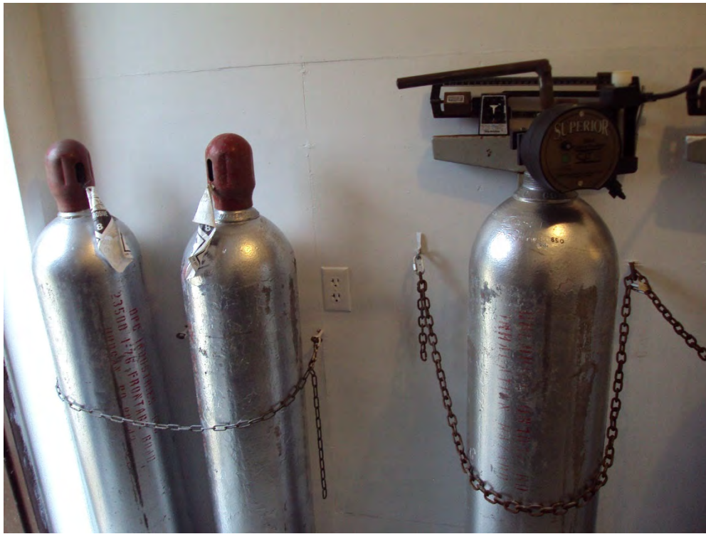
Figure 3.3: Chlorine Disinfection System
