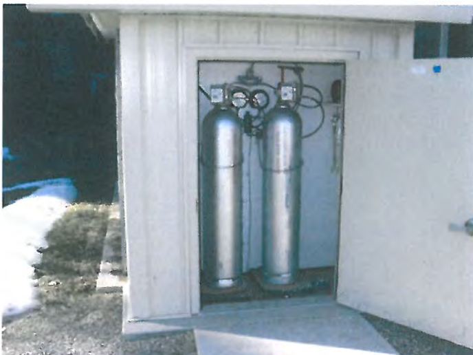
Treatment plant (TP001)
