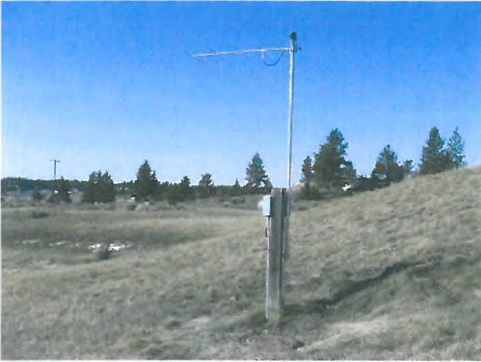
Antenna for radio controls between water level sensor in storage facility and well pumps
