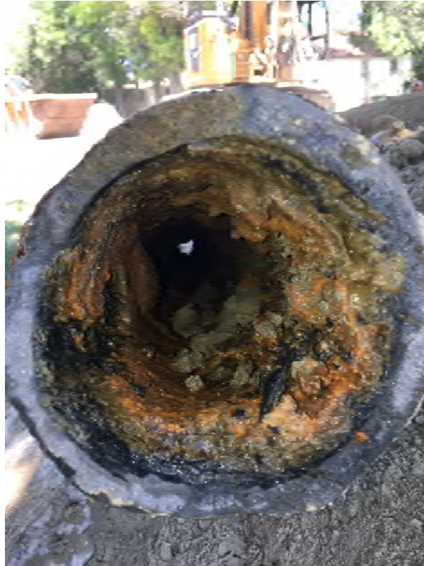
Figure 1.1: 4-Inch Cast Iron Main Condition
